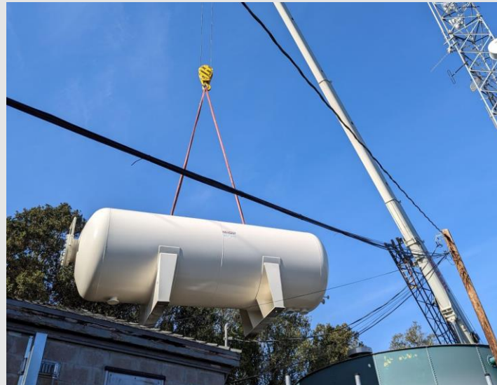
ALTA HEIGHTS PRESSURE TANK
