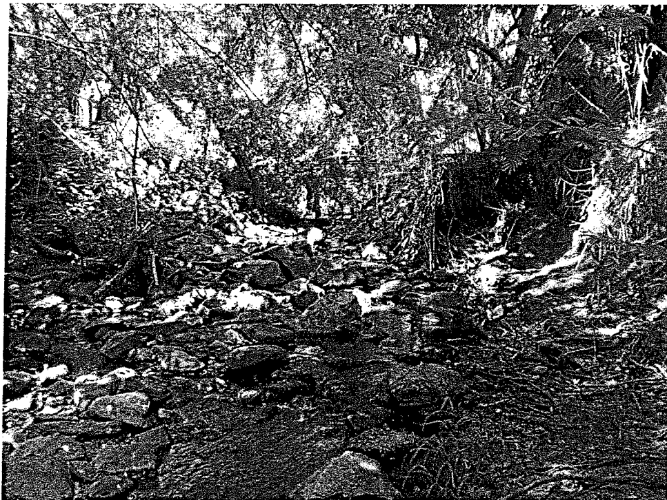
Photo 4: View looking upstream from the analyzed cross-section. Note the severe erosion along the east bank (at right), immediately downstream of the riprapped banks.
