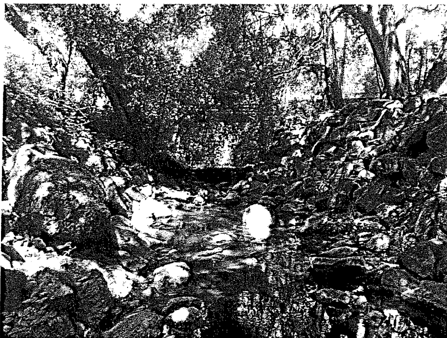
Photo 2: Upstream view along the Channel reach immediately downstream of the existing bridge, which is visible behind the tree foliage. The 2-3 ft. high grouted rock wall/grade control structure crosses the channel at the shaded center of the photo.
