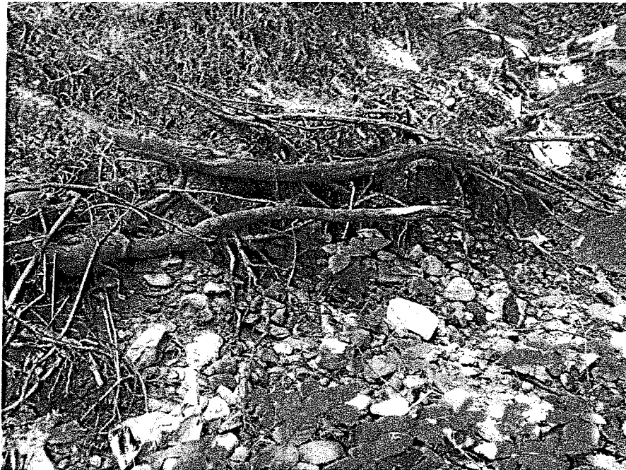
Photo 6: A close-up of the low to mid-bank zone of the west bank, immediately downstream of the analyzed channel cross-section location. Note the patch of still-intact bank soil infused with large gravel and cobble at mid-left under the tree root. Erosion of this lens of material produced the loose gravel and cobble on the lower terrace. The larger gravel-cobble component is absent in the mid-bank soils.
